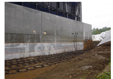
Geothermal heating system
